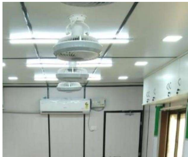
(Fan & light, AC Fittings)
